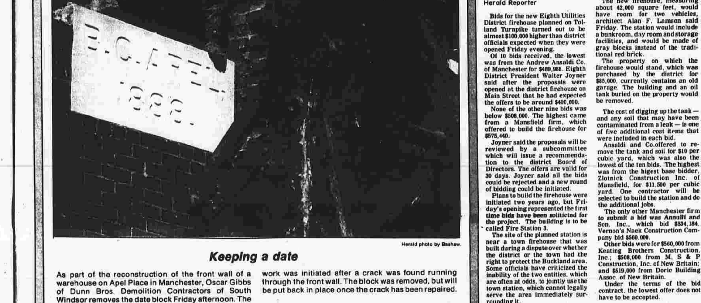
Keeping a date: As part of the reconstruction of the front wall of a warehouse on Apel Place in Manchester, Oscar Gibbs of Dunn Bros. Demolition Contractors of South Windsor removes the date block Friday afternoon. The work was initiated after a crack was found running through the front wall. The block was removed, but will be put back in place once the crack has been repaired.
